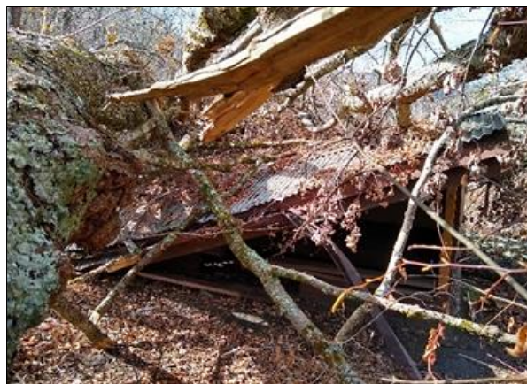
Cherry Gap Shelter ... Crushed!
