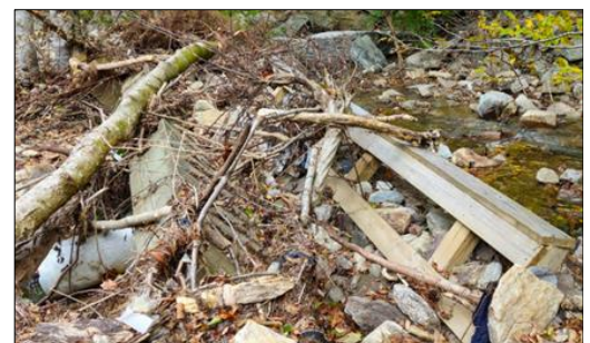
Missing Footbridge just South of US19E
