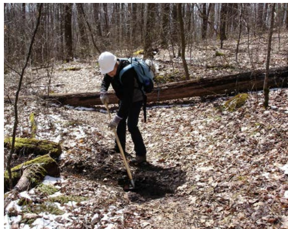
Terry cleans out a water diversion near the blowdown ½ mile south of shelter
