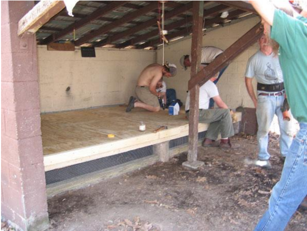
Installing the Abingdon Gap Shelter Sleeping platform, photo courtesy of Carl Fritz
