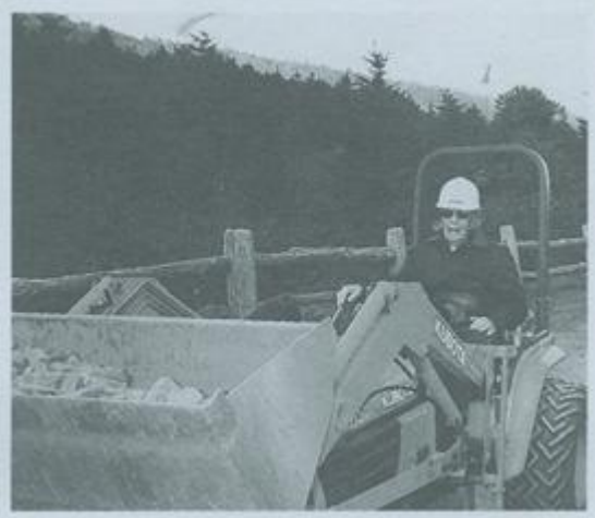
Frank Oglesby, age 89, operating front-end loader during Round Bald A.T. relocation project in 2000 (photo by Joe DeLoach).
